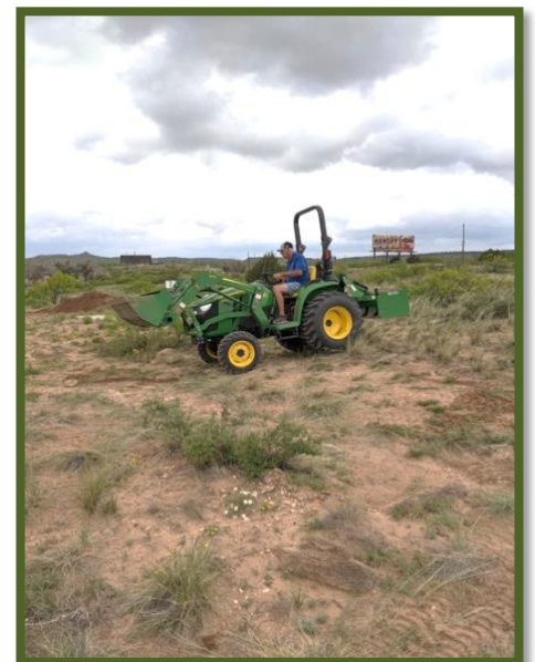
Volunteers working to build a walking path at Five Mile Park in May 2021
