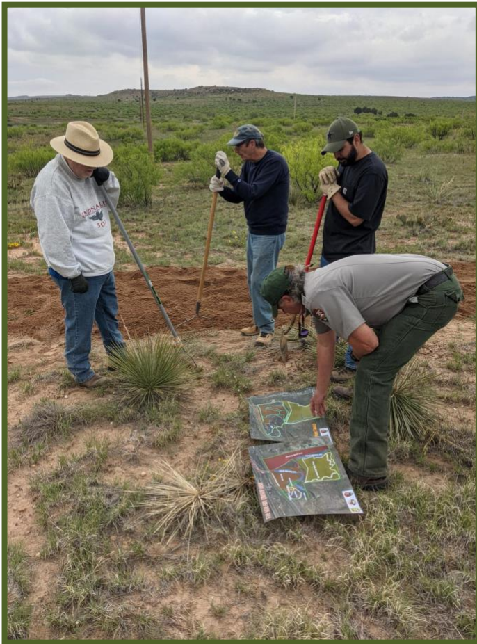
Volunteers working to build a walking path at Five Mile Park in May 2021
